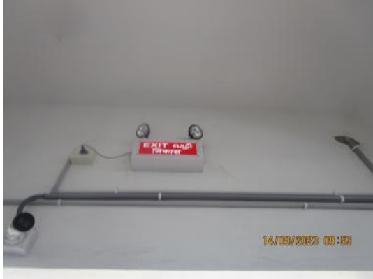
Emergency exit illuminated light system.JPG
