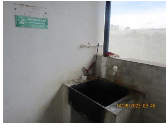
Hand wash basin.JPG
