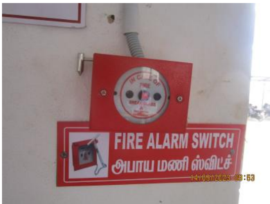
Emergency call point.JPG
