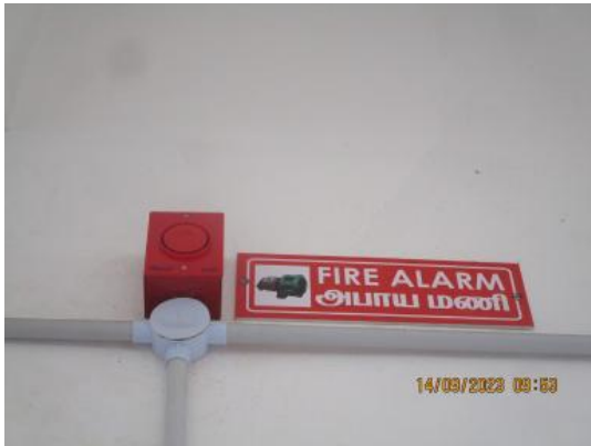
Emergency alarm system.JPG
