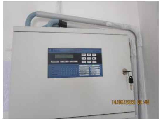
Fire control panel.JPG
