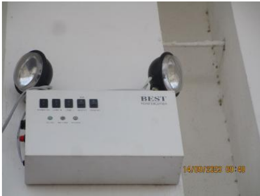
Emergency light system.JPG
