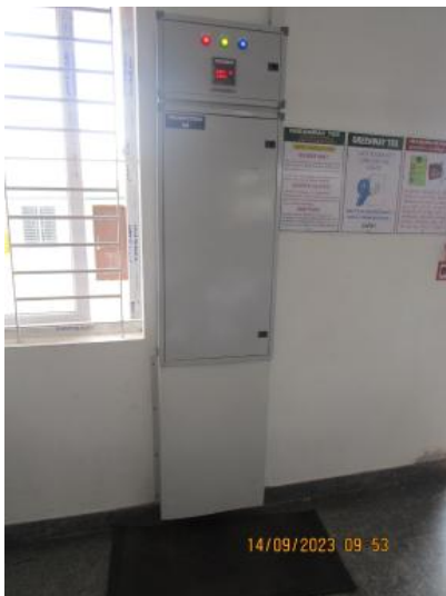
Electrical panel board.JPG
